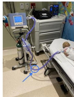
Vent Circuit has too much "rainout" or condensation in the tubing causing an obstruction to flow. Drain the circuit back into the heater chamber.
